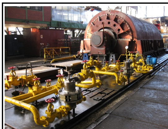
Fig. 1. General view of the turbogenerator
