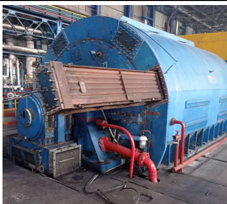
Fig. 2. General view of the turbogenerator gas cooler
